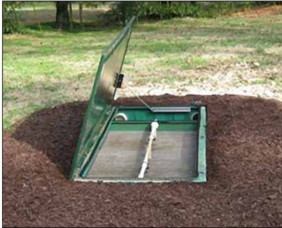
This AX20-RTUV with Ultraviolet Disinfection, engineered by Kevin Davidson, is the first to be approved by the North Carolina Department of Water Quality for a surface discharge permit.
